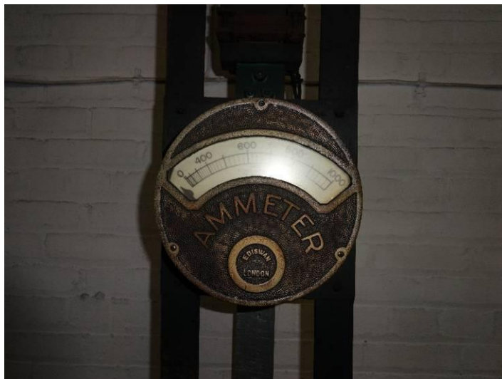
Detail of an ammeter at first-floor level. The ammeter is used to measure the current in a circuit.
