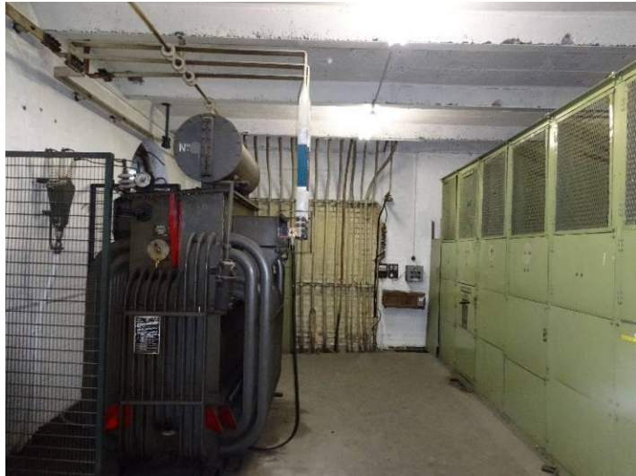
Interior of ESB transformer sub-station, looking east
