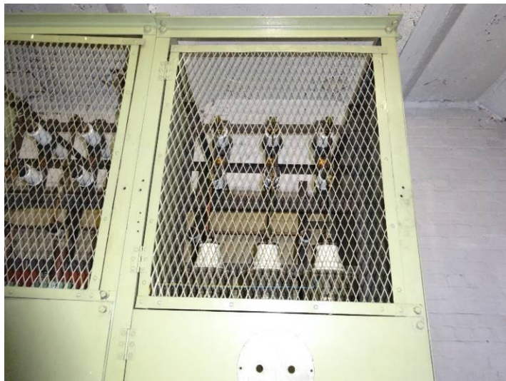
A detail of the 1940's equipment at ground-floor level
