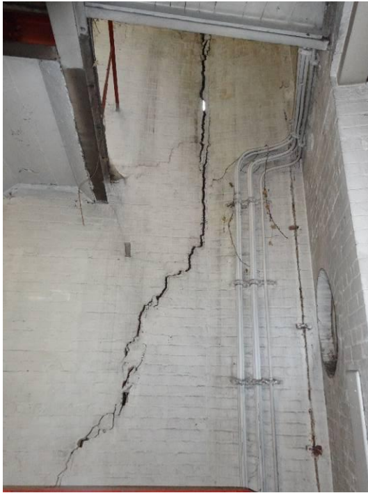
A vertical crack at the west end of the southern rear wall
