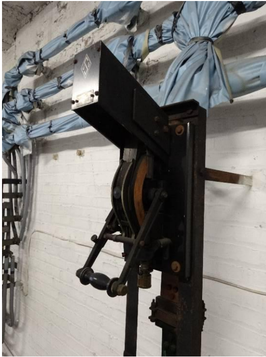
Detail of one of the many switches at first floor level
