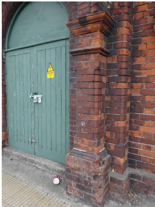
Brick pilaster with pedestal and moulded cornice to south of entrance door
