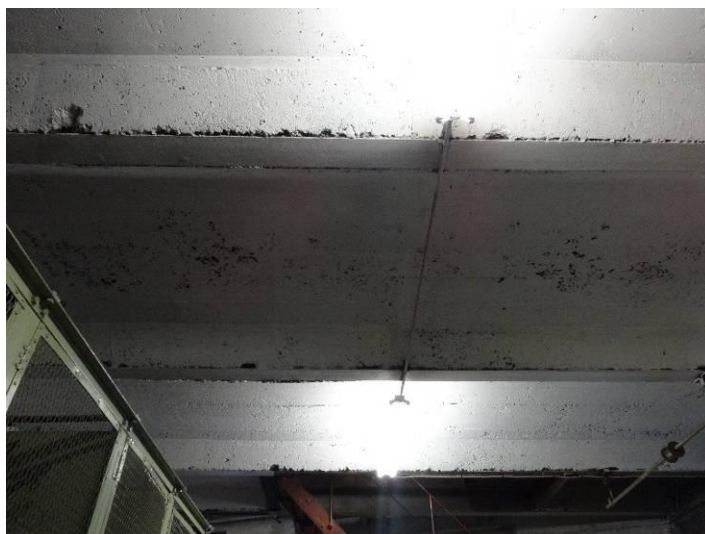
Detail of the underside of the concrete floor at first-floor level. The concrete floor is supported by steel joists.
